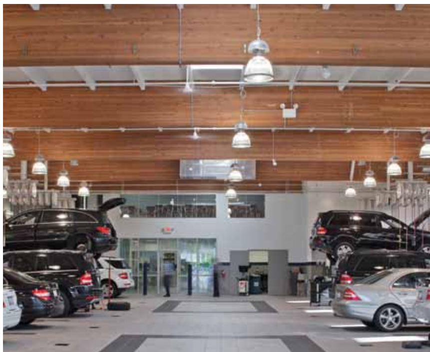
LEDs were used mostly where the “world can see them,” meaning CMH fixtures were the workhorse in the service area.
